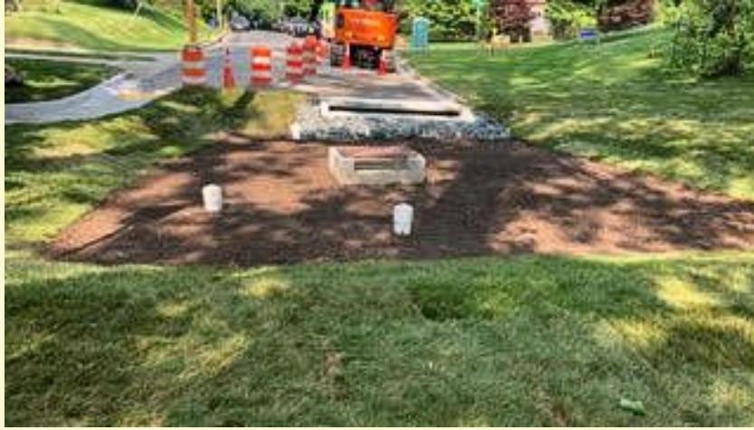
During construction, looking north toward Melbourne Ave. Notice the drop from street height down into the bioretention area and the subsequent rise in height to help keep water from heading into Three Oaks. (MCDOT photo)
